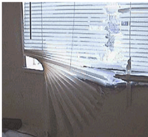
RIGHT: Impact damage to window blinds and sill.
